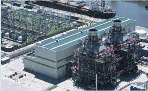
Combined Cycle Power Plant
